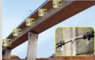
Fiber sensors mounted on bridges
