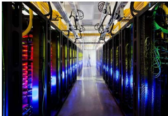
Google data center
